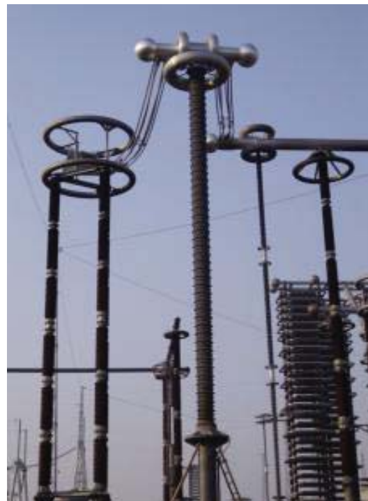
Figure 1 800kV DC ECT
