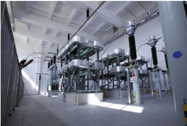
Figure 4 TBS of 500kV UPFC Project in Suzhou, China
